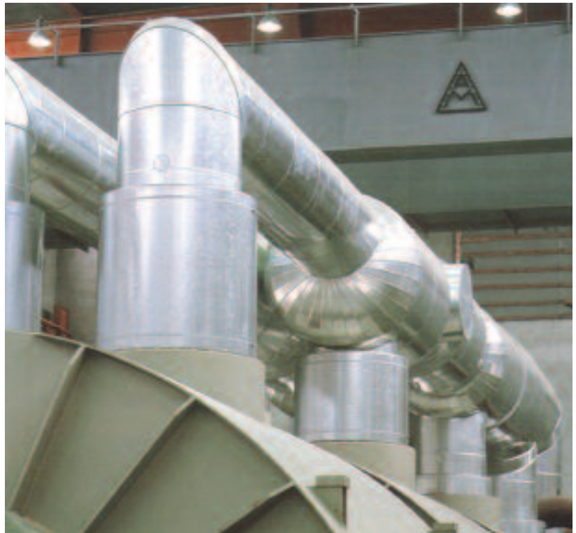
Lamella Mat used to insulate ducting - thickness of insulation maintained under cladding load
